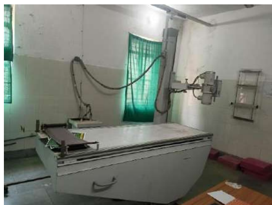
Glimpse of X-Ray machine installed
